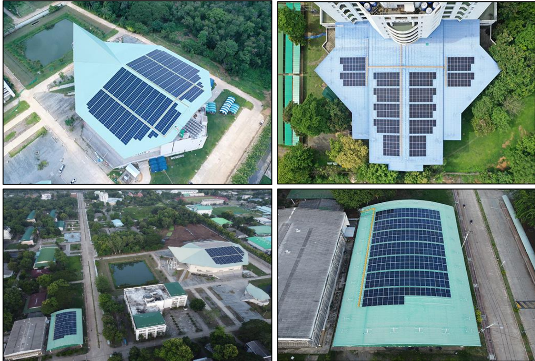
Roof solar panel
